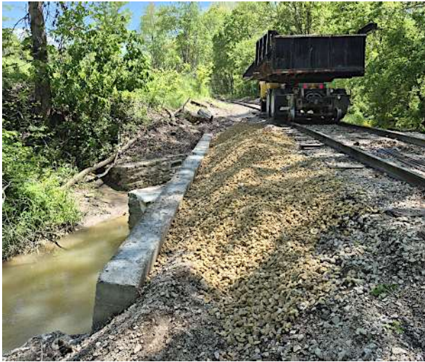
This is the finished project. Our hi-rail dump truck is in the background. It was used to transport the gravel. The bed swivels sideways so the gravel could be dumped to the side.
